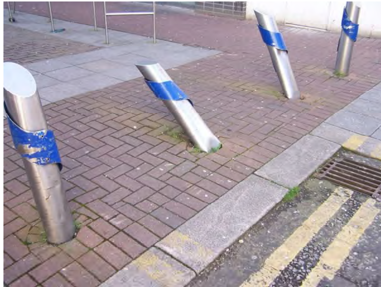
Figure 6: Route 5 impact point showing damaged bollards
